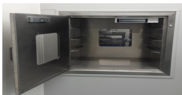
Figure 12: Example of Pass through Hatch
