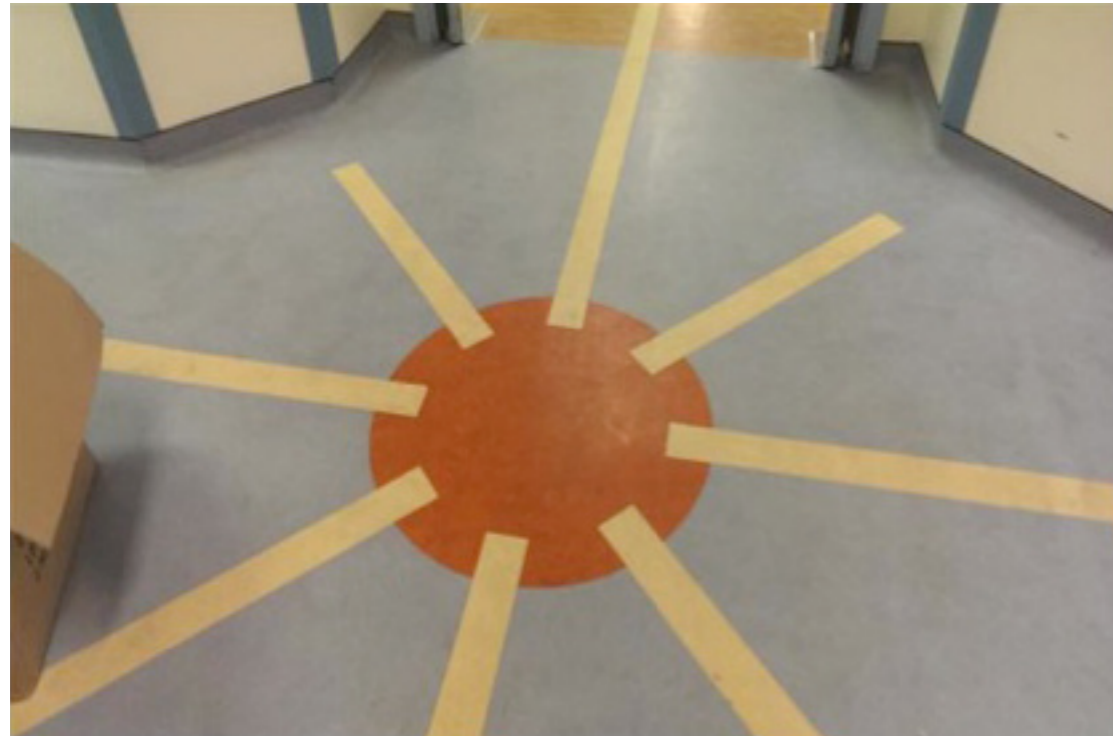
Flooring – before (note troublesome blocks of colour)
