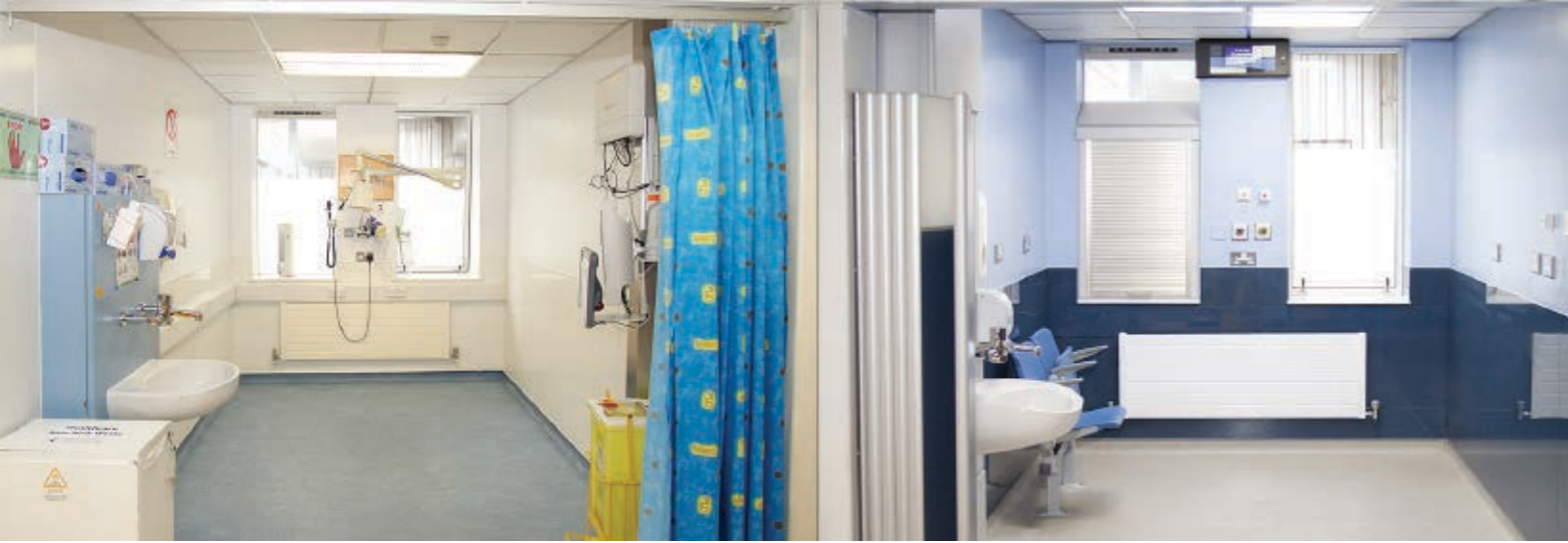
14 Before (left) and after (right) images showing retrofit of ED bay in St. James's ED.
