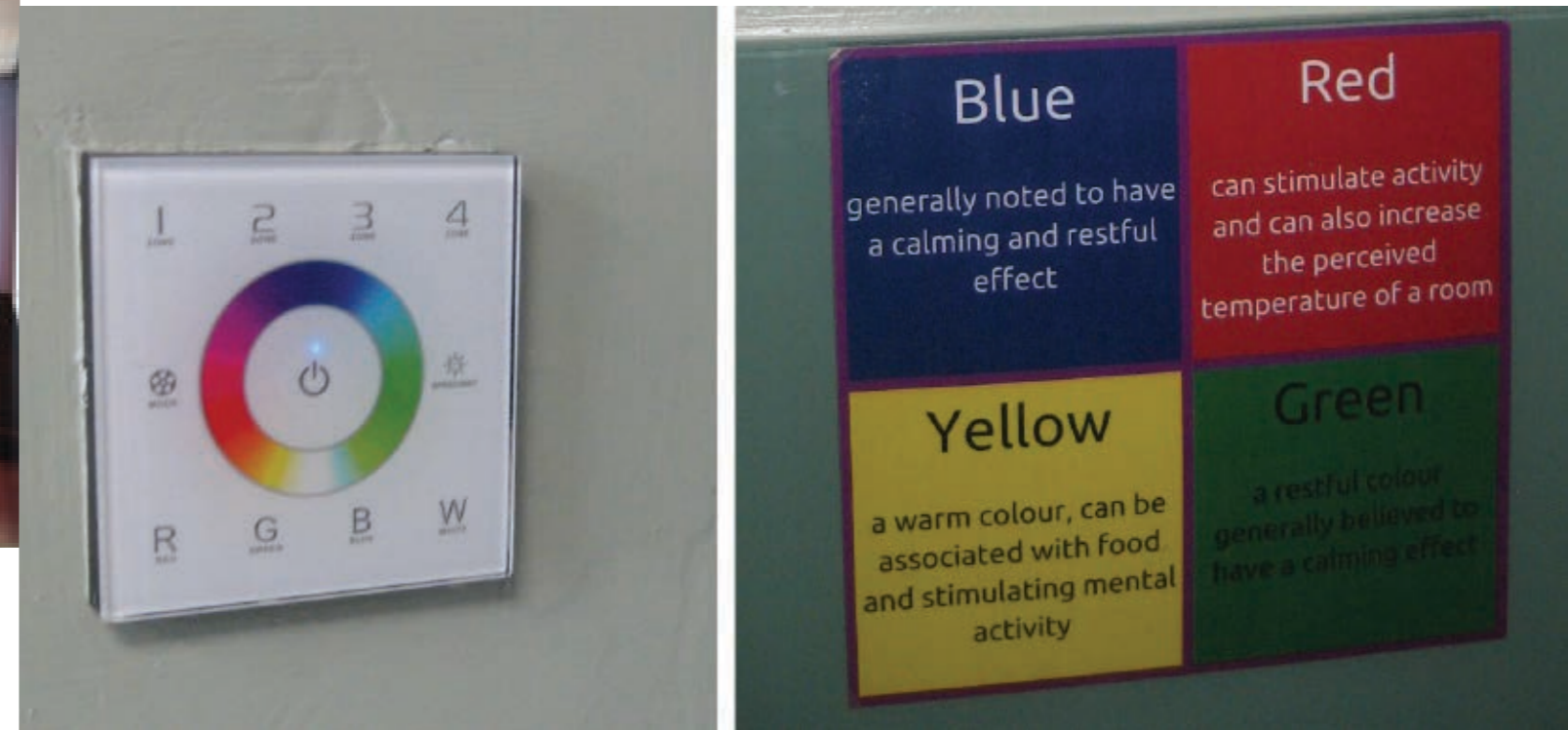
02 Lighting control panel (left) and lighting information (right) fixed adjacent to control panel. ED bay, St James's Hospital, Dublin, Ireland
