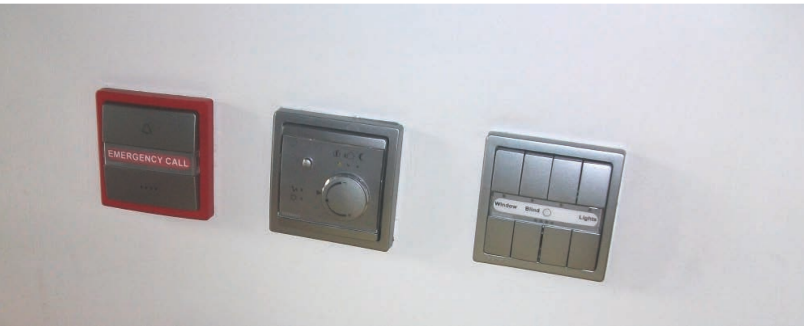
09 Emergency call button and light switches.
